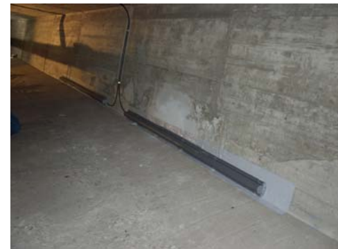
Dual 2-meter Optical Strands inside the bridge deck
