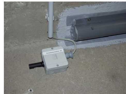
Flood detector near an Optical Strand
