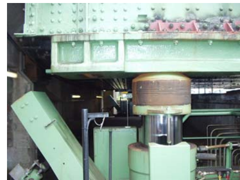
Lifting of rear end of the bridge to remove the bearing before rotation
