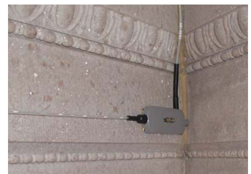
Close-up of splice box at one end of Optical Strand.
