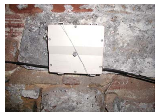
Crack watcher X-Trigger on the subbasement level.
