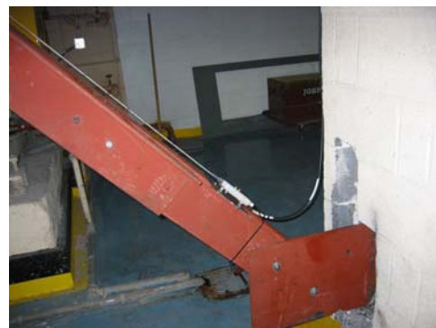
Optical Strand on a beam at a technical floor
