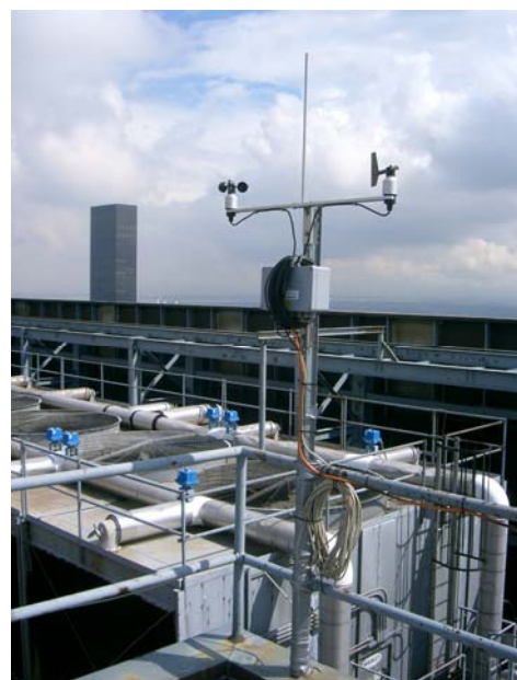
Wind gage (Speed and direction) on the roof
