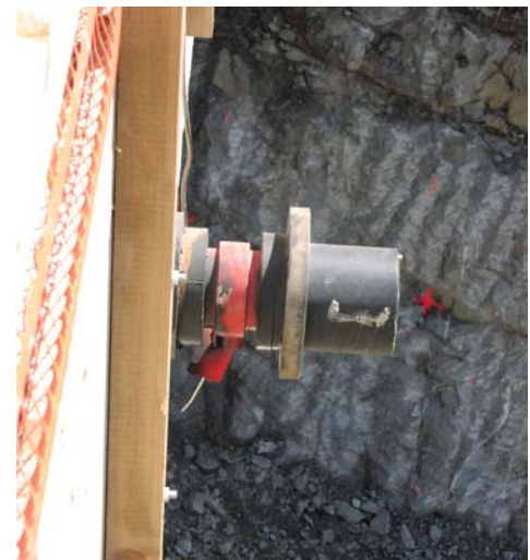
Load cell on an anchorage head
