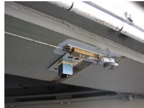
Optical Strand splice box equipped with a micrometer
