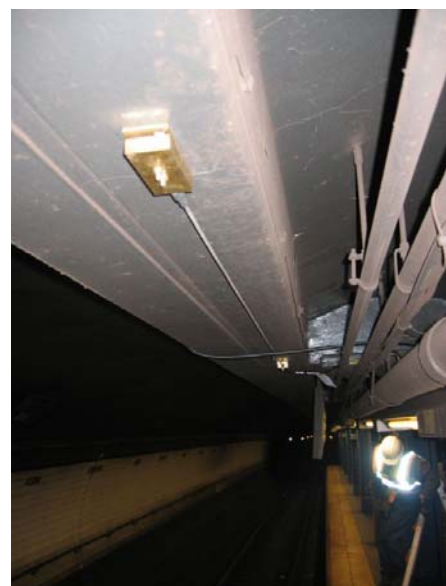
Optical Strand on a beam
